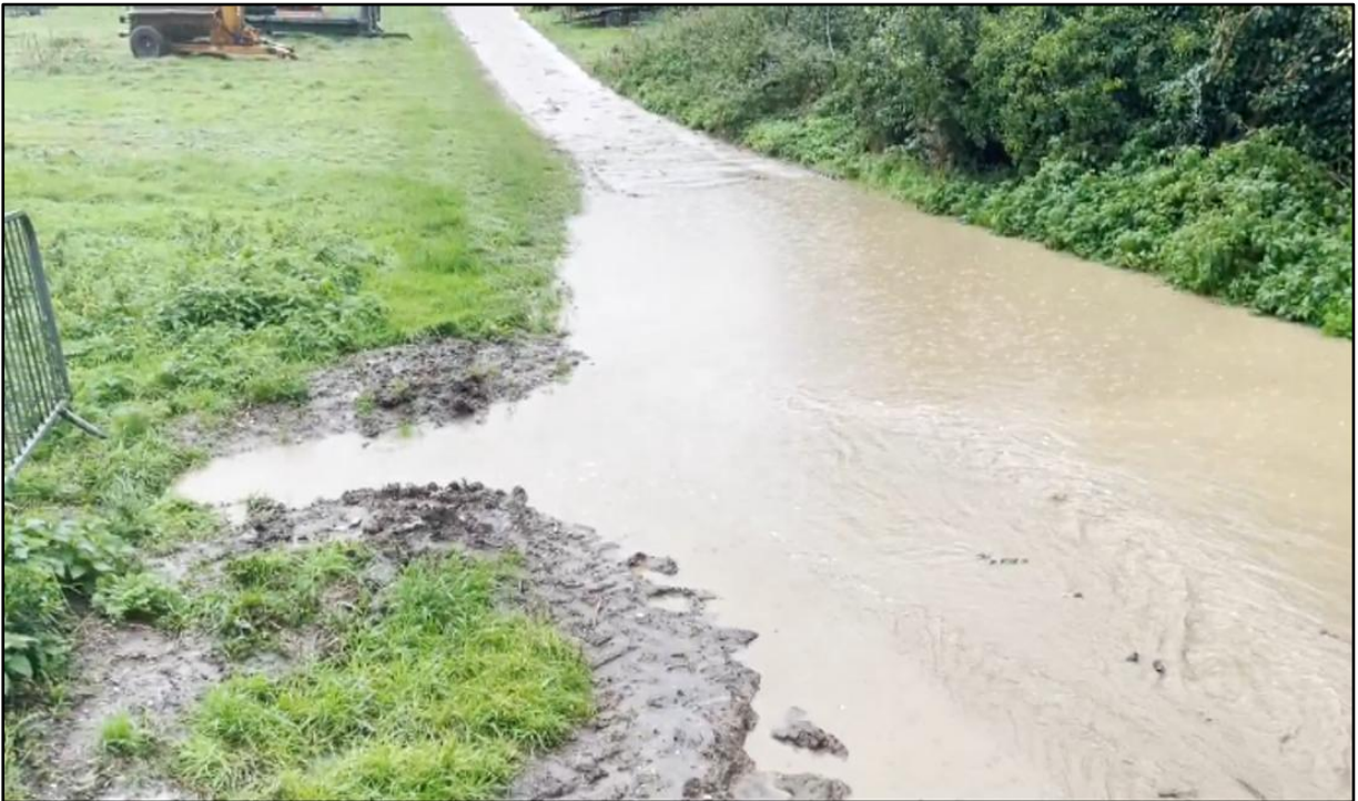
Image 5 - Surface water runoff from Witten's Meadow construction site towards Mow Hill (photo looking southwest)
