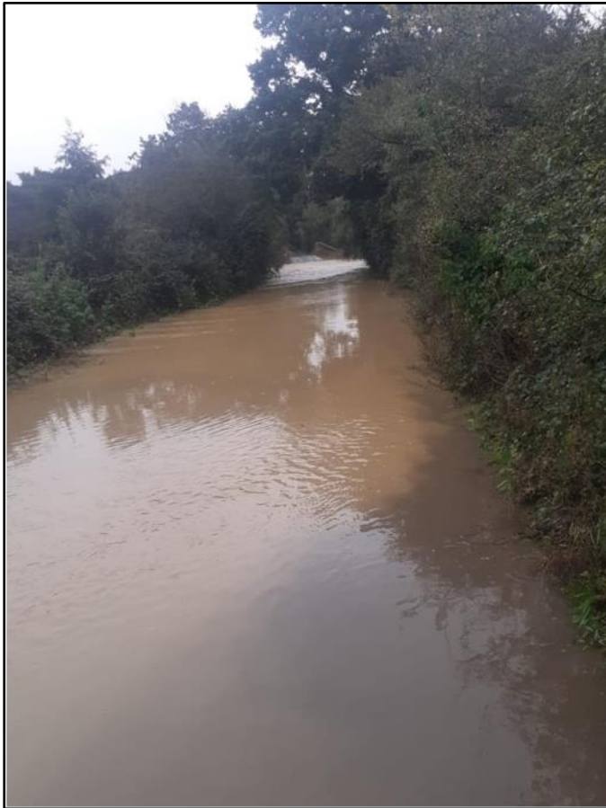
Image 3 Flooding at Boot Street road bridge
