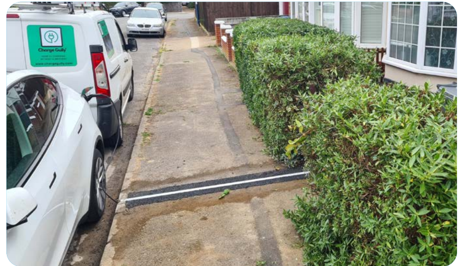
Image 10: A photo of the Charge Gully installation being used to charge a vehicle.
