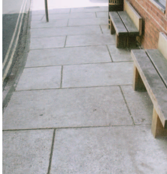
The size of the bays in relation to the proportions of the footways and the pattern of the expansion joints should be an important consideration
