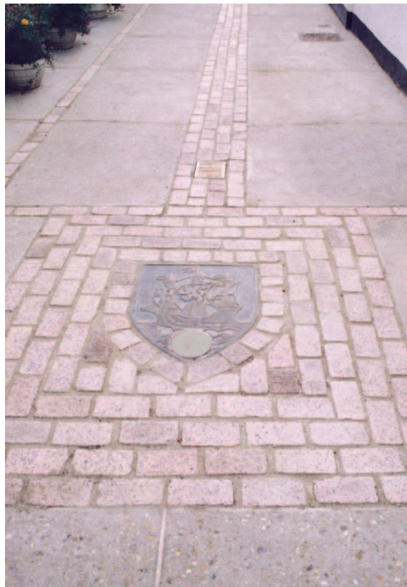
In situ concrete and pink granite setts were traditionally used in Aldeburgh and were specified for the resurfacing of Town Steps
