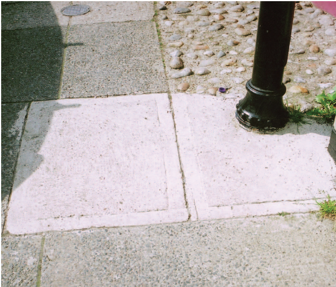
A tamped surface with a 'frame' around the edge is not an acceptable finish in historic areas
