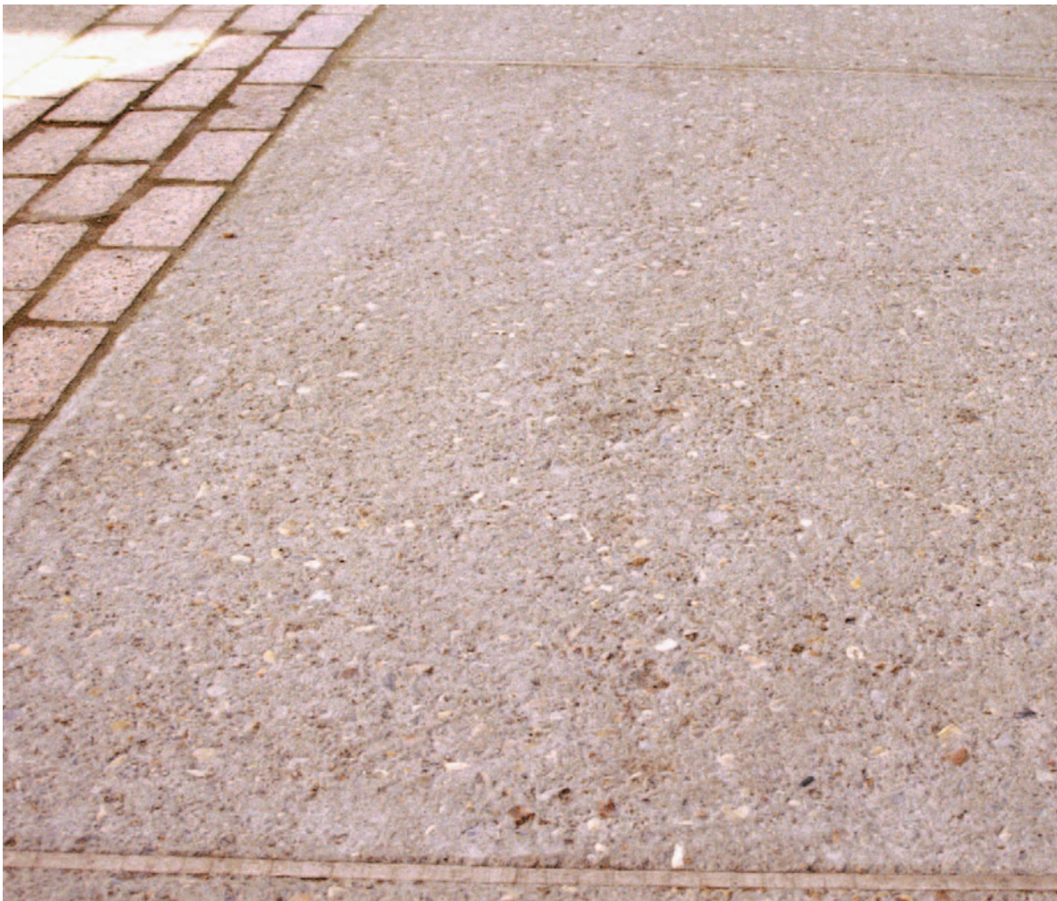
The finish on this concrete was achieved with the use of a 'scabbling' machine
