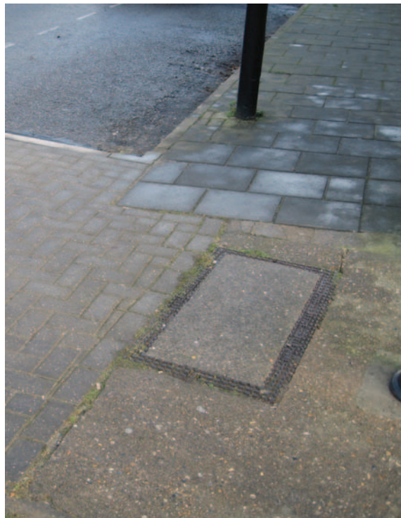
Concrete paviors may be convenient to use but in many instances they will not enhance the street scene
