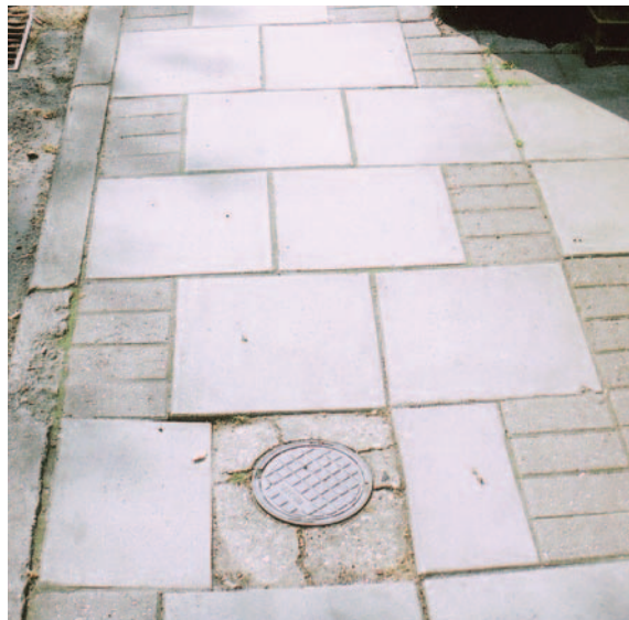
Infilling using concrete paviors is no longer an acceptable practice
