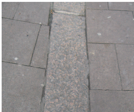
Small pieces of cut slab and infilling with concrete should be avoided.
