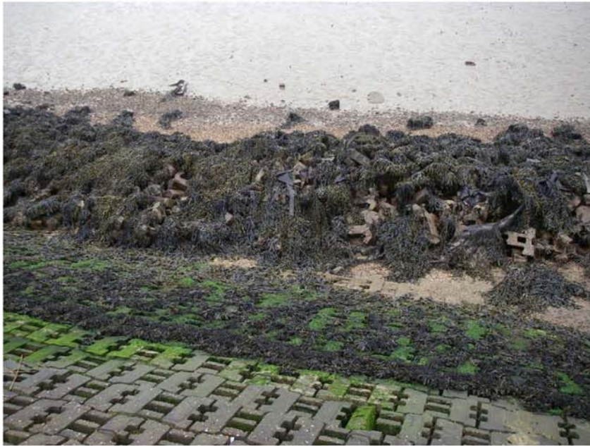
A low energy attenuation/saltings protection bund constructed from Ankalok remnants, this can be found along the Hazlewood frontage of the Alde Estuary.
