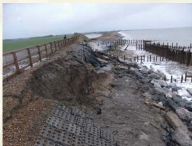
Coastal Path Erosion at Bawdsey after the December surge tides
