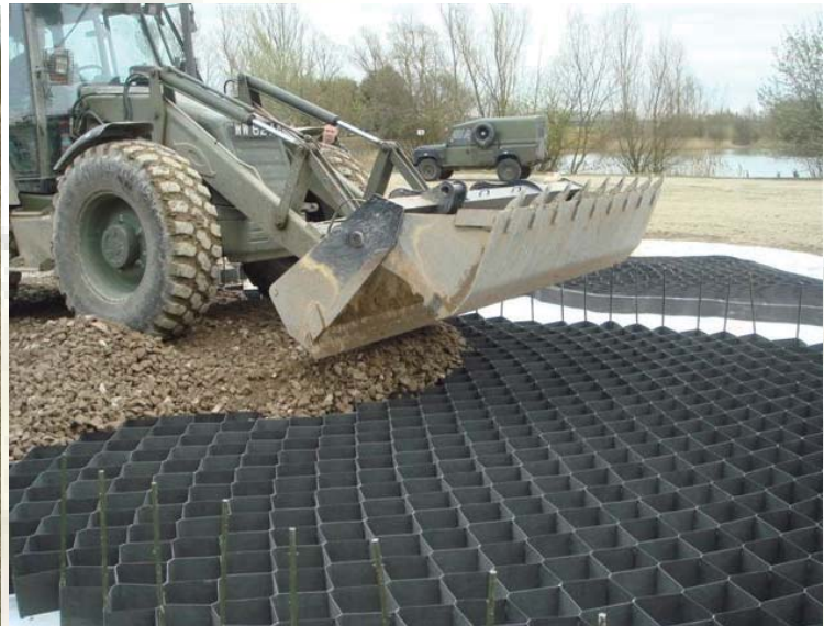
In extreme circumstances the above system could be implemented, it is incredibly strong and durable to allow construction traffic to pass over it. Large areas can be covered in a day.
