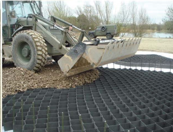
In extreme circumstances the above system could be implemented, it is incredibly strong and durable to allow construction traffic to pass over it. Large areas can be covered in a day.
